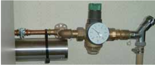
Installation of the AquaKat on the water supply before the pressure reducer of the oven
