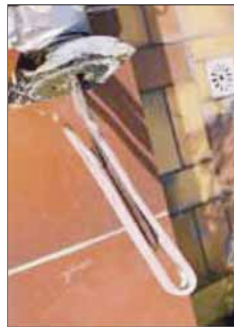
D These limescale deposits were, however, according to SBZ professional tester Karl Maierthaler, “totally soft” and “could easily be removed with a jet of water”.
